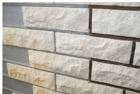
The installed clinker façade tiles along with grouting joints on the insulating panel
